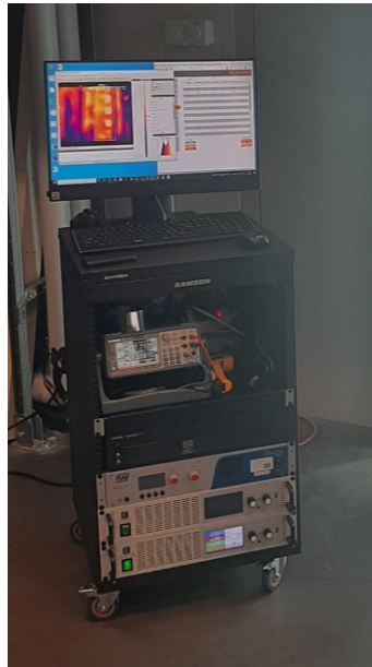
Figure 4 Smart Rack #01 setup for in-suite monitoring
