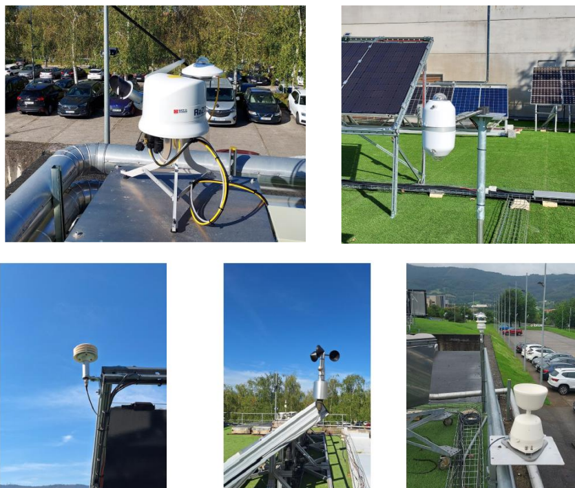
Figure 5-3: Meteorological sensors at TecNALIA outdoor facilities
