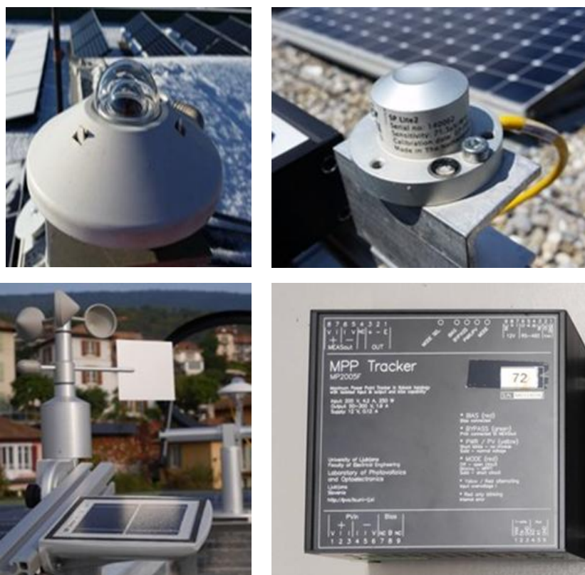
Figure 3-3: (Top row and bottom left) Examples of the radiometric sensors and wind gauge available on the CSEM monitoring platform, and (bottom right) a detailed view of the monitoring/MPPT unit.
