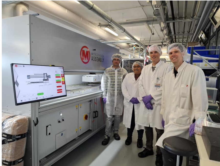
Figure 2: Final verification after the installation in CEA.
