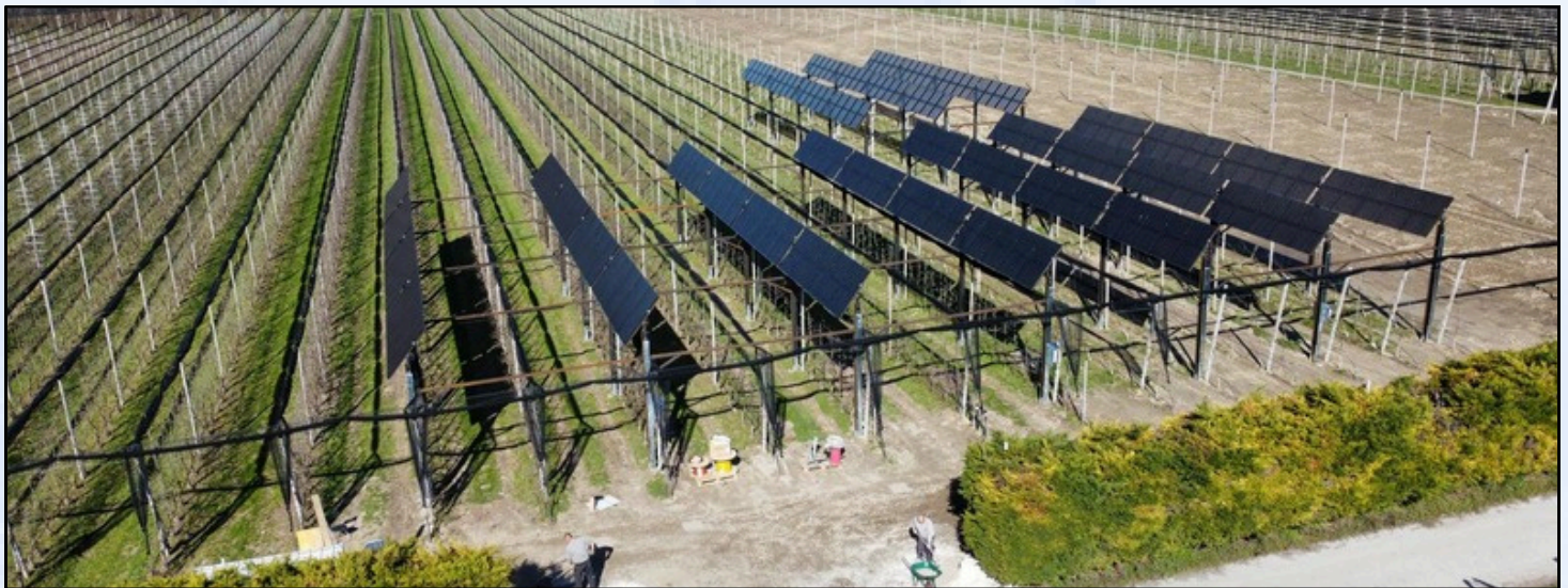
▲ A pilot Agri-PV site in Bolzano (Italy), Symbiosyst project
